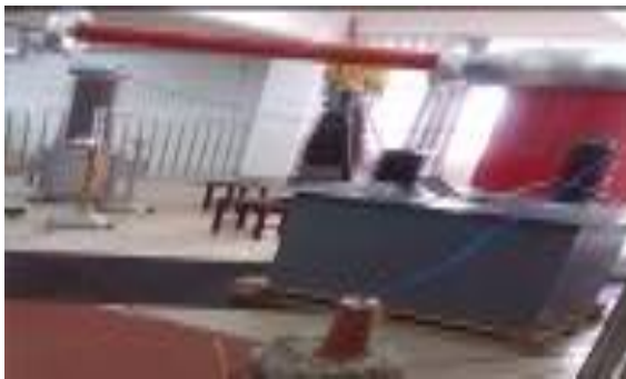
Fig. (3). Experimental devices on 0.4kV/10kV power transformer PD detection.
