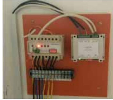
Figure 6 sub control device
