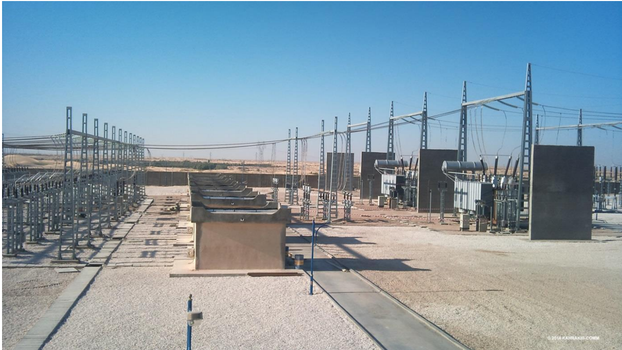
Fig. (1). Components of the national distribution network.
