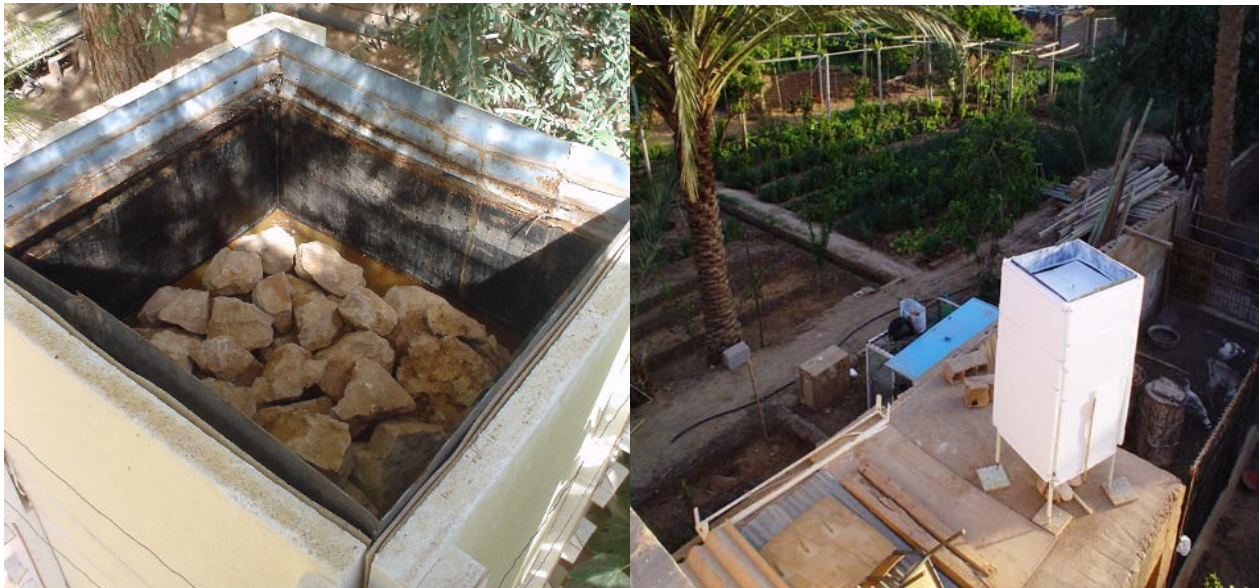
Fig. (4). The evapo-reflective roof.
