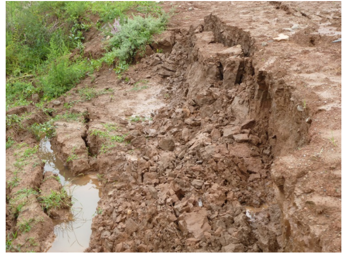
Fig. (5). Ponding water at the trailing edge of landslide.
