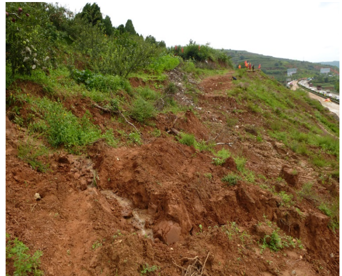
Fig. (6). Water on landslide surface.
