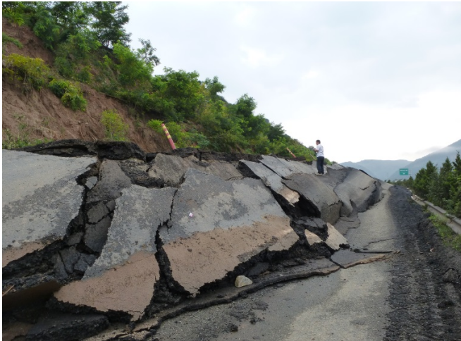
Fig. (7). Pavement bulging at the leading edge of landslide.
