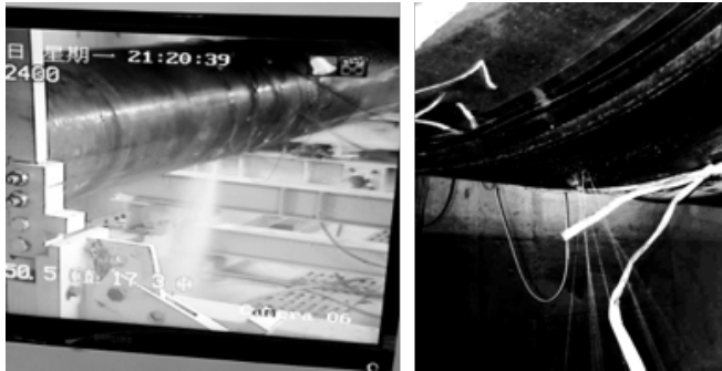
Fig. (6). Sample leak condition.
